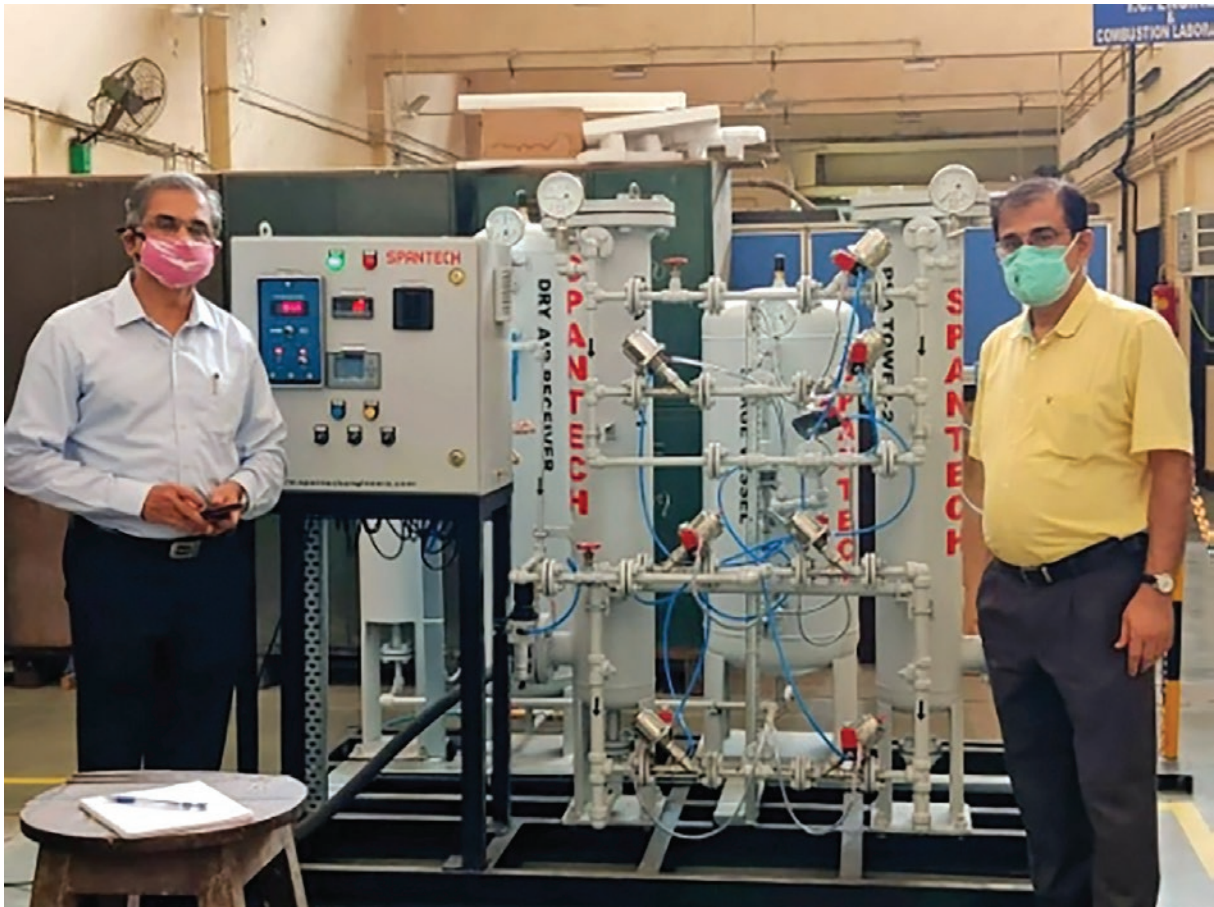
Indigenous system to produce oxygen using PSA unit
