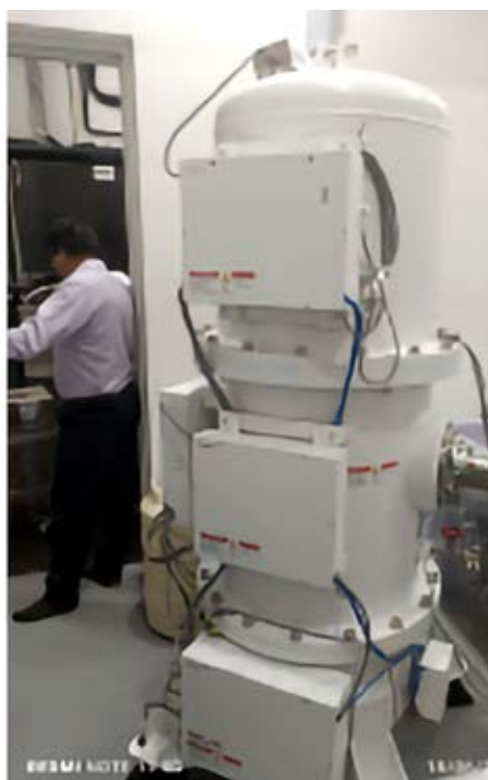
High Tension Tank
